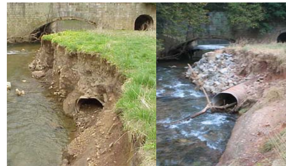
(a) (b) Figure 2. Streambank loss in front of George Washington’s Headquarters between 2001 (a) and 2004 (b) resulting in exposure of a sewer line.
